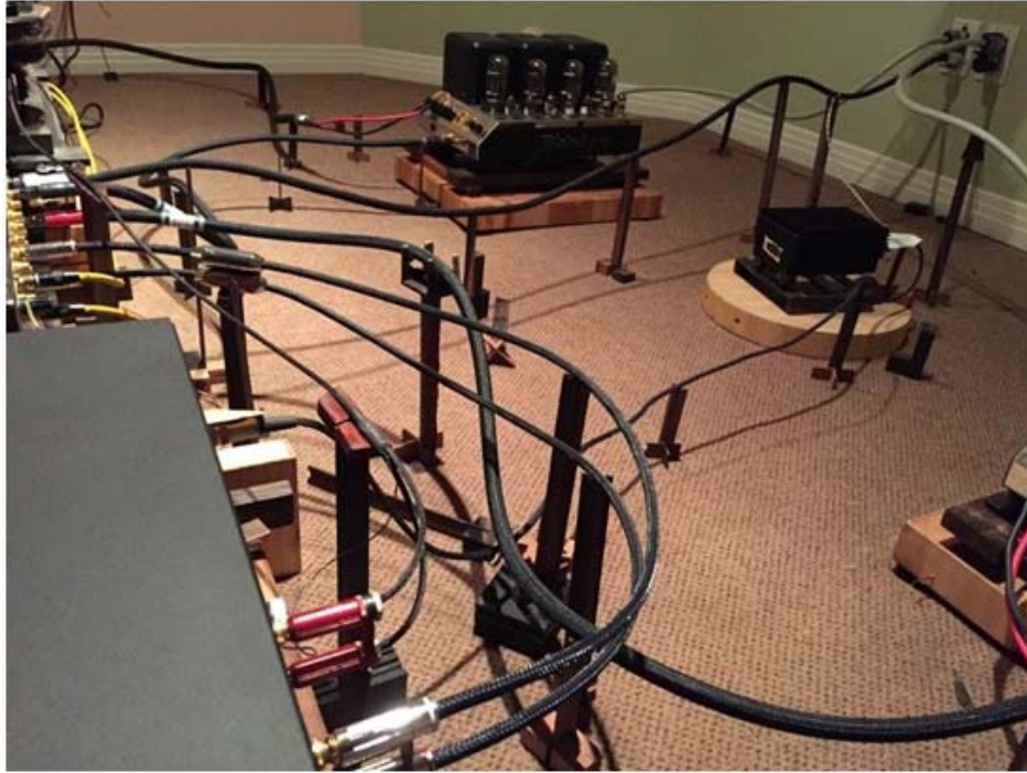
(Cable Risers deployed at the Leevite Residence)
